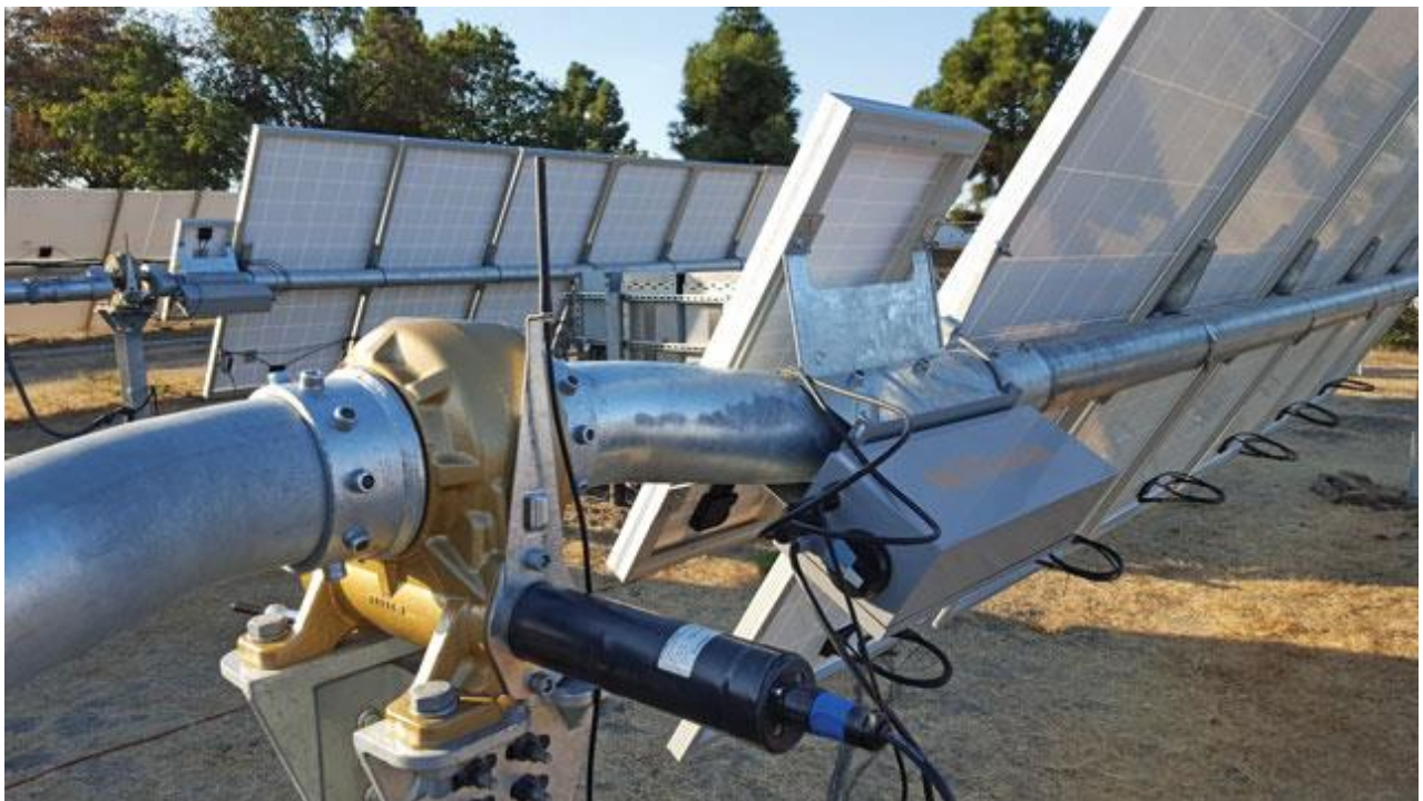
Figure 1: Single-axis tracking array (source: NEXTracker)
