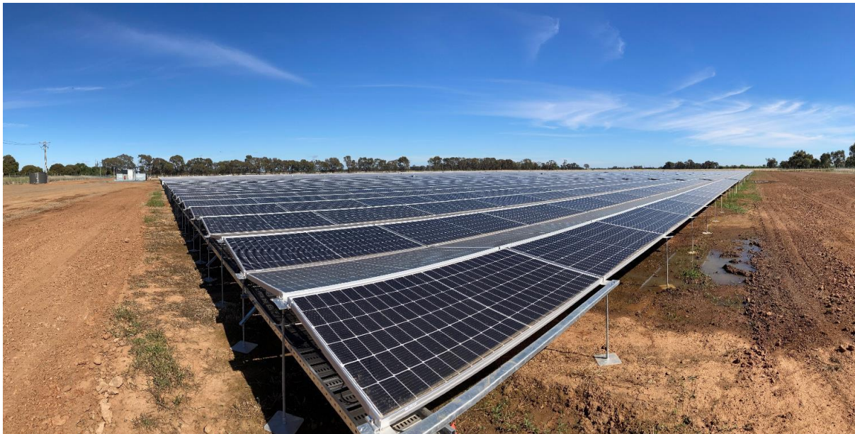
Figure 2: Belectric mounting system (source: ITP Renewables)
